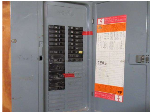
200 amp breaker box located behind pool equipment building.
