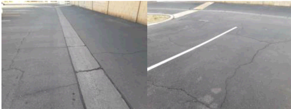
Sealcoat without Crackseal
