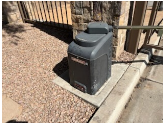
These are LiftMaster CSw24UL swing gate operators (8/28/2020).
