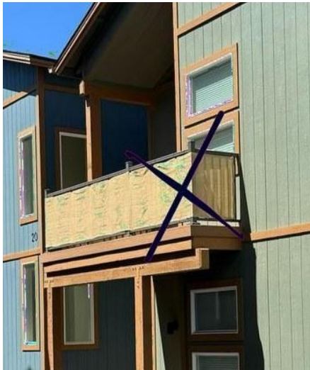
✗ NOT ALLOWED — mounted outside, hardware visible
