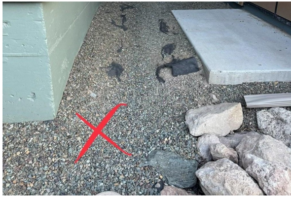
X NOT ALLOWED — worn path, exposed weed barrier
