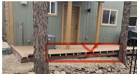
✗ NOT ALLOWED — incomplete skirting, exposed framing
